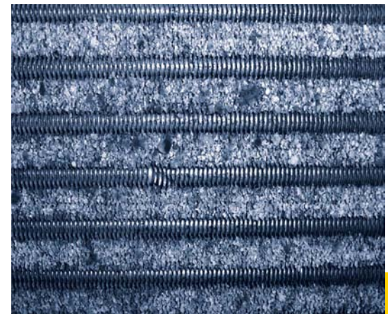
Biofilm growth in a cooling coil
