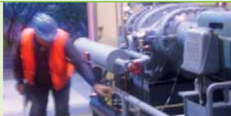
Plant room of an ammonia refrigeration plant room at a cold storage facility in Victoria
