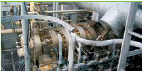
Part of hydrocarbon refrigeration system for making liquid ethylene at temperatures as low as -100^{\circ}\text{C}
