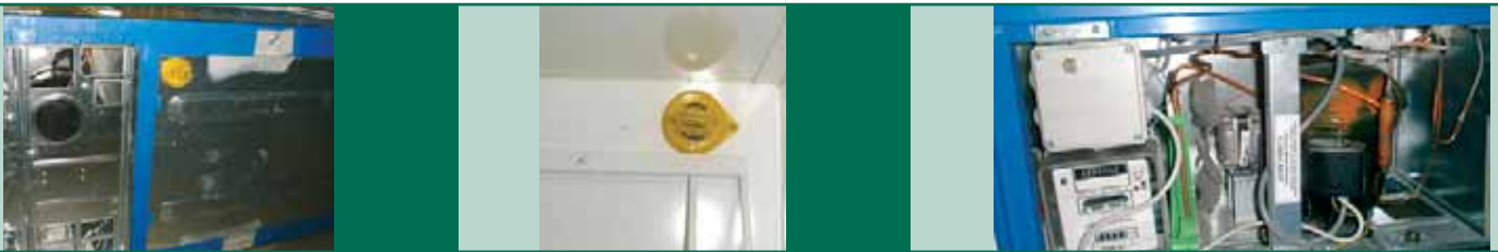
(L-R) Data loggers inside and outside the Unilever ice cream cabinets, and an electricity meter placed on the bottom of the cabinets
