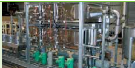
Ethylene-propylene cascade system used for recovery of petrol vapour at -80^{\circ}\text{C} . It uses hermetic compressors (green items visible at the edge of the unit)
